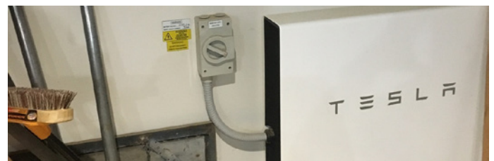
12.4kw Tesla Battery System with back up function to enable use during power outages.
