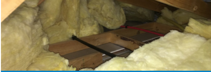
A number of areas were identified that were missing insulation. These will be rectified by the builder.
