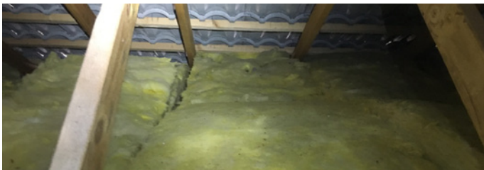
R6 insulation installed correctly in most places
