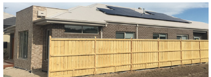
5kw Solar systems installed with excellent northern orientation
