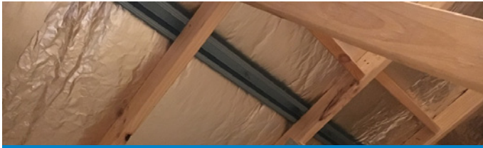
Anticon Blanket R1.3 under colorbond roof. As well as assisting insulate the home it stops condensation and dust entering the roof space.
