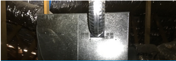
Gas ducted heating unit installed in the roof space
